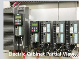
Electric Cabinet Partial View
